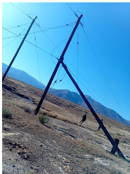
Picture 2. Old Electrical poles destroyed by extreme weather
