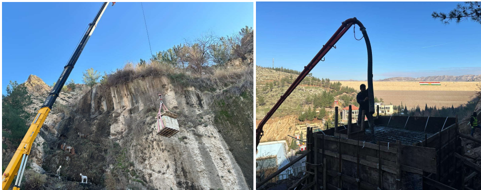
Fig. 10: Transporting materials and fittings and casting concrete for the water tank using a crane and a pump poster.
