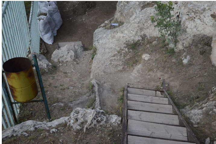
Fig. 4: Pre-existing situation. Unsafe stairs, no stairs, deteriorated handrails, and bins on the west side of the Charsteen Cave.
